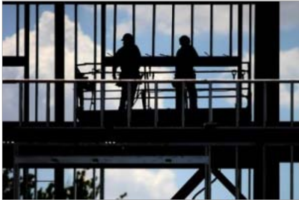
Crews from Timberlake Construction work to build the new St. Eugene Catholic Church on Hefner Road between Pennsylvania and May avenues. (Photo by Brent Fuchs)
